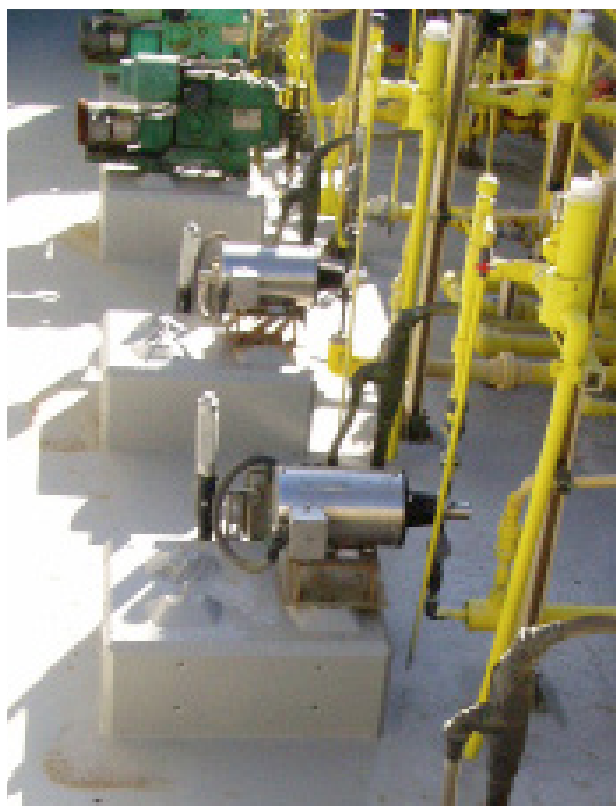
The compact Tuthill design allowed easy replacement of diaphragm pumps in this 12.5% NaOCl installation.
