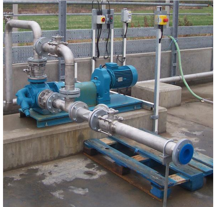
Tanker Offload Installation
